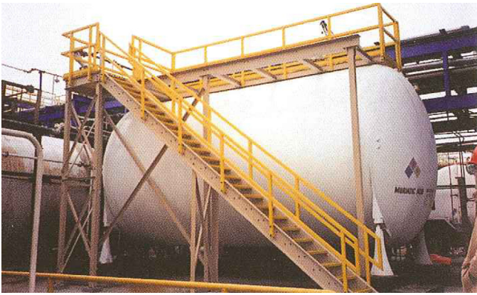
SAFRAIL™ system in a chemical plant.
