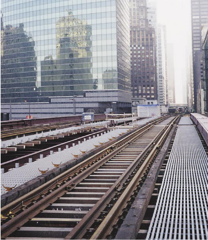
Chicago Transit maintenance walkways alongside elevated train tracks constitute one of the largest fiber glass grating installations in history. The project used DURAGRID® T 5000 2" with a custom polyester resin.
