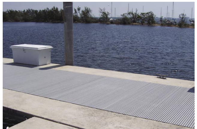
DURAGRID® T-1700 pultruded grating was used to replace wood planks on a large walkway at Dinner Key Marina in Miami, Florida. The grating allows for easy accessibility to utilities below the walkway and will not rot like the previous wooden walkway.
