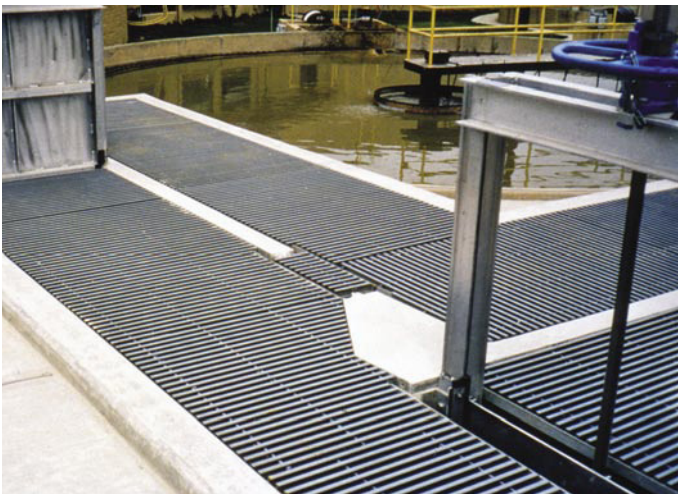
Low maintenance fiberglass grating trouble free operations for the covers and walkways in the Lakewood, Colorado Wastewater Treatment Plant Headworks. DURADECK® I-6000 1-1/2" was used.
