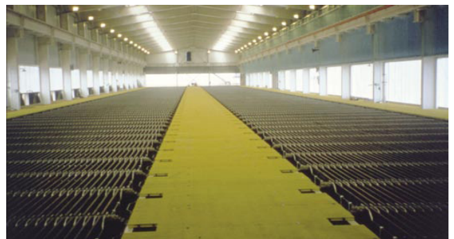
Cooper processing facilities such as the Ammonia Leach/Solvent Extraction Electrowinning plant for Minera Escondida Limitada in Chile found DURADECK® I-6000 1-1/2 to be the perfect solution.
