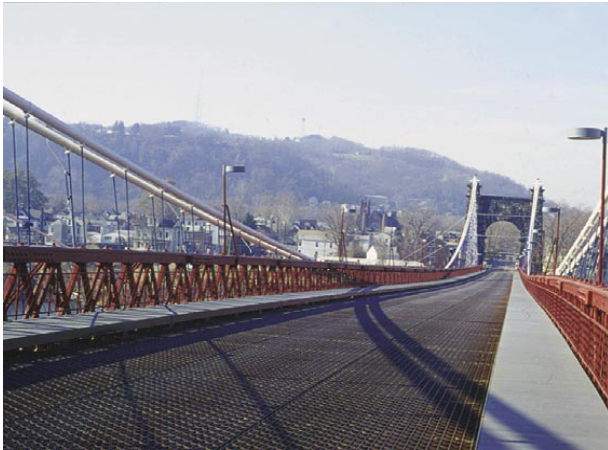
Eight-thousand square feet of DURAGRID® I-4000 1" pultruded grating replaced steel side-walks on this bridge in West Virginia.
