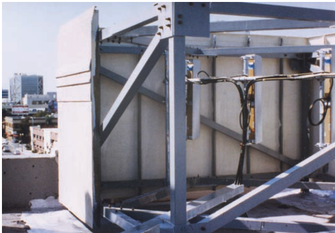
EXTREN® fiberglass plate and structural shapes were used for cellular shielding and were made to match the style and appearance of the appearance of the Santa Ana Historical building.
